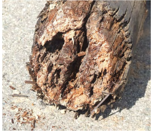
Photo B-6. Pole Split inside a Pole
